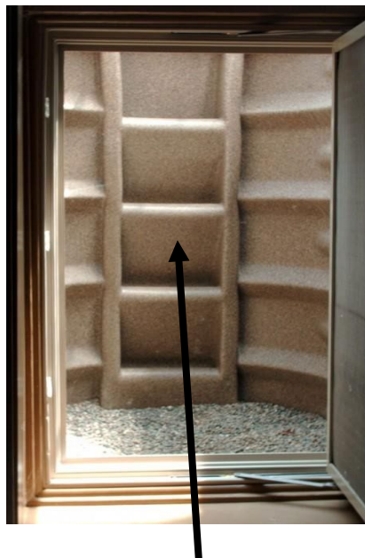
Looking from the basement through the egress window into the egress well.
